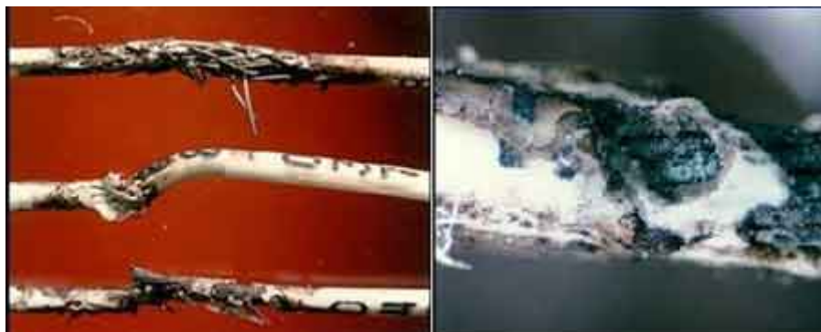
Wiring showing insulation breakdown emanating from failure at hot stamp mark sites, taken from an in-service US Air Force aircraft
